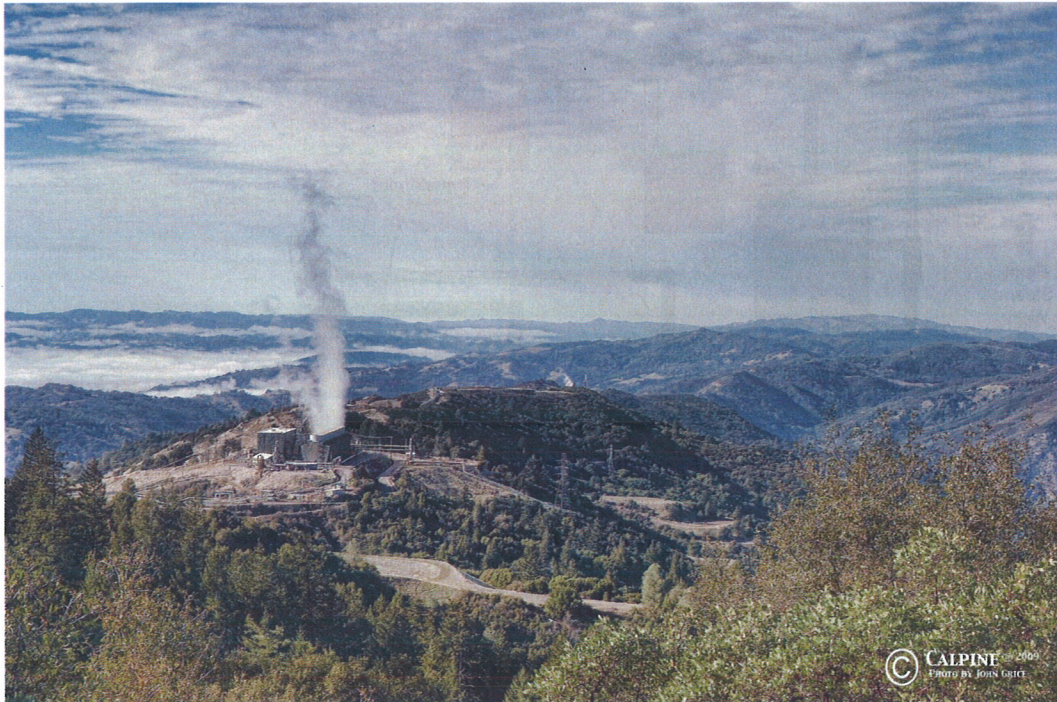
FIGURE 3.2 Ridgeline Unit 7 and 8 Power Plant (rated at 69 MW) in the left foreground at The Geysers in California. The turbine building, housing the two turbine-generator sets, the operator’s control room, and various plant auxiliaries are on the left. The evaporative cooling tower with steam emanating from the top is on the right of the main complex. The beige pipelines along the roads (with square expansion loops) are the steam pipelines that gather the steam from the production pads and bring it to the plant. A high-voltage transmission line (denoted by lattice towers) is in the middle foreground of the picture. SOURCE: Calpine.
